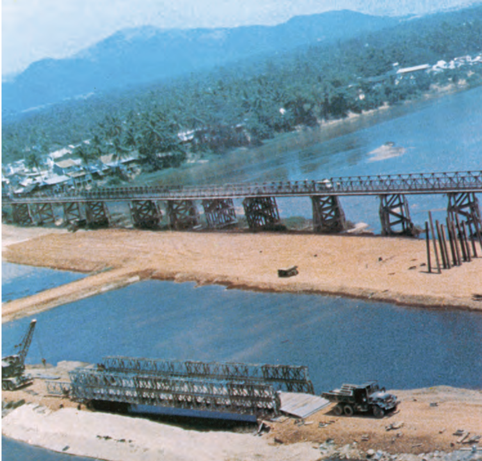
Troops of the 84th Engineer Battalion build the new Bong Son Bridge.
